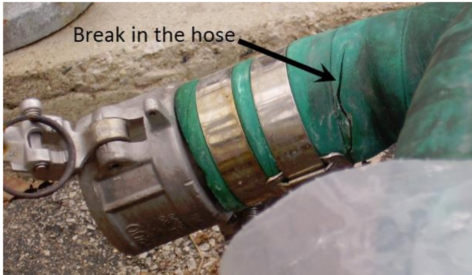
Figure 1. Photograph of the failed hose showing the location and appearance of the break.
